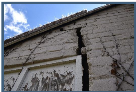
West end gable failure - north crack.
