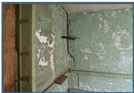
North wall separating from interior dividing wall.
