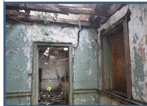
South wall separating from interior dividing wall.
