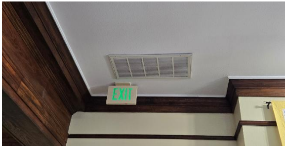
Fig.II.258 An air return duct for the larger HVAC system.
