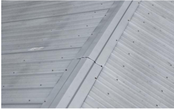
Fig.II.68 Ridge cap tops the roof. Undetermined if foam closure was used below the cap assembly.
