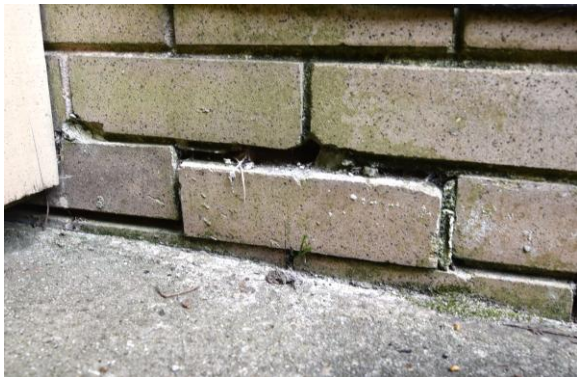
Fig.II.39 Dislocated brick on north elevation at grade due to water invasion and freeze/thaw cycle.
