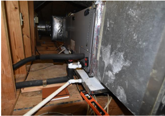
Fig.II.253 5-ton air handler located above young adult reading room.
