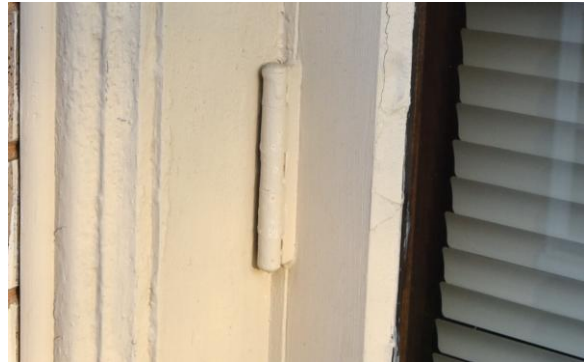
Fig.II.204 The windows are not operational due to overpainting of seams and hinges.
