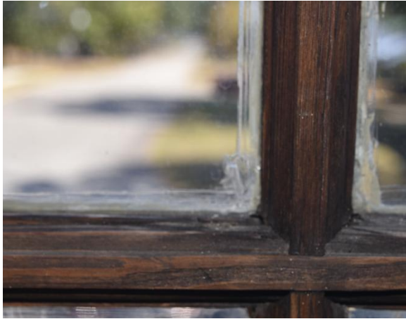
Fig.II.211 Silicone chalk was applied to the interior on many of the windows.
