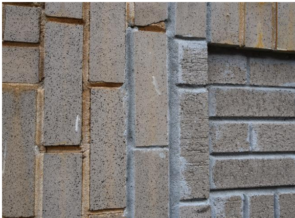
Fig.II. 31 Patching (repointing) to the water table brick above the ADA doorway used unsympathetic Portland based cement mortar.
