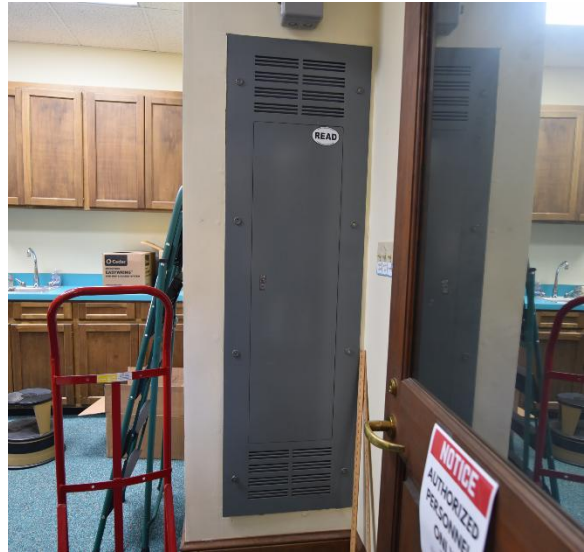
Fig.II 239 Main electrical panel is located in the librarian's office along segment of west wall.
