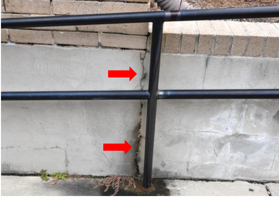
Fig.II.98 Complete wall failure due to poor drainage is underway.
