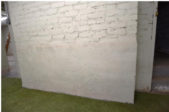
Fig.II.5 Lower portion of interior basement walls covered with skim coat of concrete.
