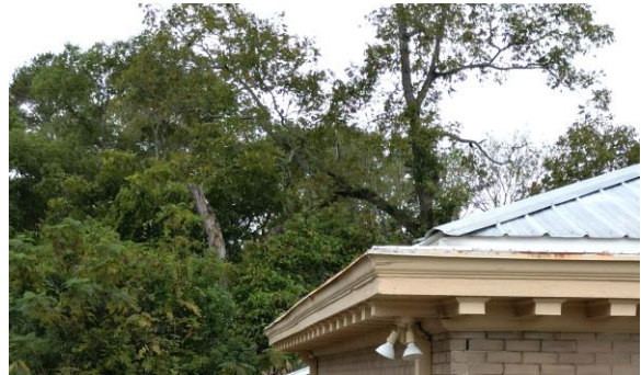
Sec. I/Fig. 53 Two trees in the building rear are threatening the structure.
