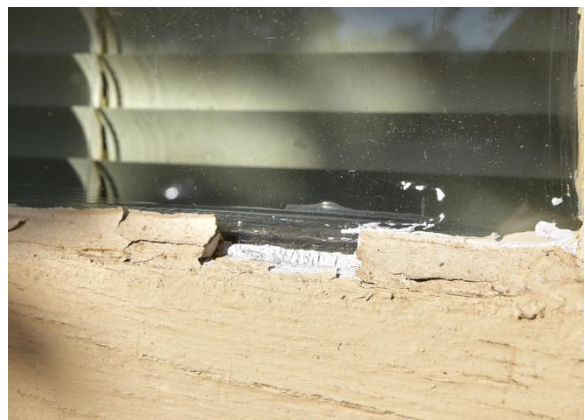
Fig.II. 210 Many windows have failing glazing (putty seal on exterior).
