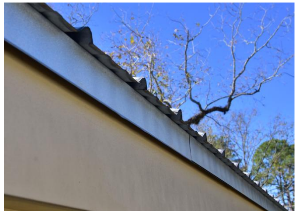
Fig.II.89 Several roof facets have no drainage system, only an overhanging drip-edge.
