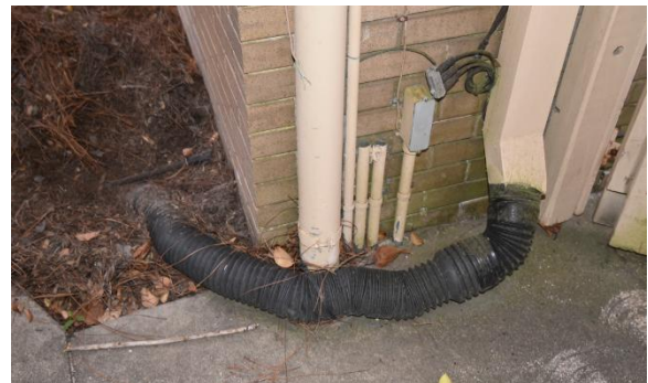
Fig.II.93 At the northeast corner, the ground drain directs water into small yard area lacking effective drainage.
