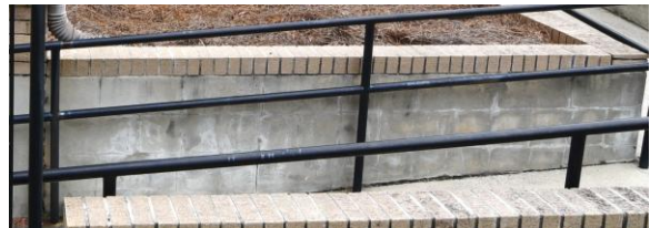
Fig.II.97 The white lines along the mortar are evidence of excessive moisture seeking a "way out."
