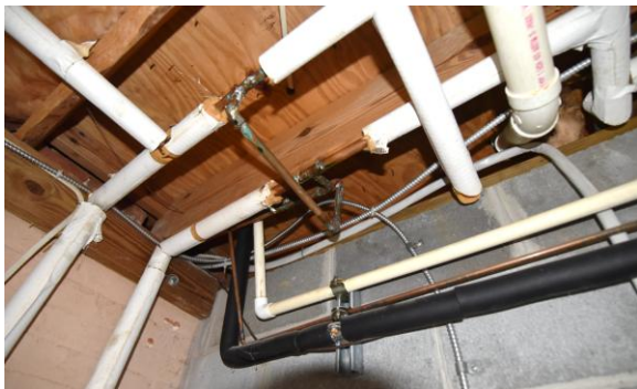
Fig.II.259 Waste lines are PVC and supply lines are copper, nicely insulated in most places.
