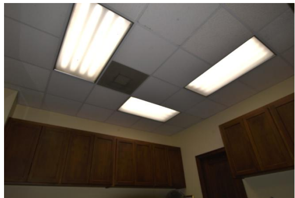
Fig.II.246 Fluorescent fixtures are used throughout the 1990s Addition.
