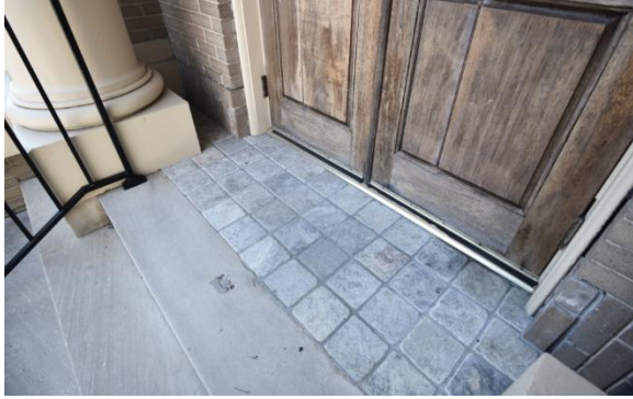
Fig.II.228 The top stair landing is finished with non-historic tiles.
