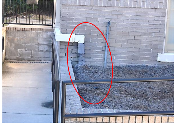
Fig.II.96 Rain runoff on south end of east elevation is trapped by ADA ramp and wall.
