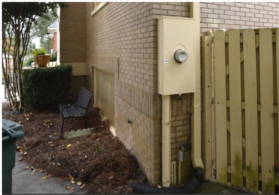
Fig.II. 238 Electrical meter in northeast corner of building.
