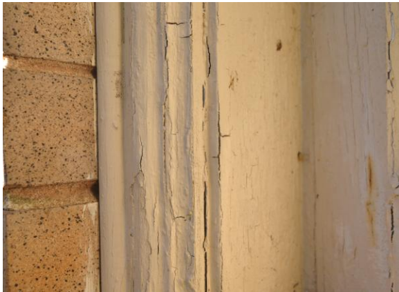
Fig.II.207 Various types of paint failure was observed.
