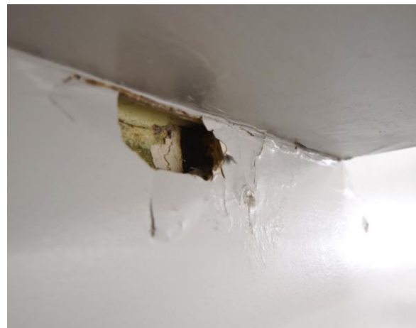
Fig.II.108 Extensive gypsum board failure below entryway in basement.
