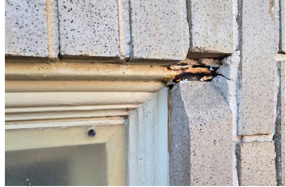
Fig.II.40 Fractured brick and iron jacking above basement window east elevation.
