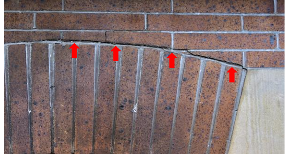
Fig.II. 159 Mortar failure above segmented arch on north fireplace.
