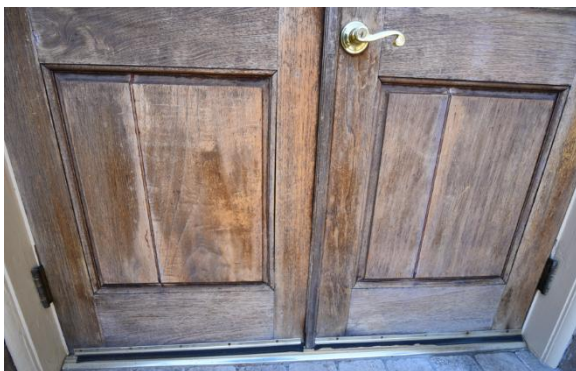
Fig.II.182 Finish on exterior of main doors has degraded and needs restoration.
