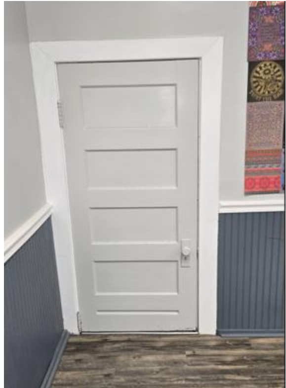
Fig.II.180 Note how door has been dramatically shortened at the bottom. A strong indication that the floor was raised from original height and doors cut down to fit.
