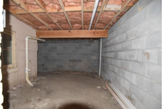
Fig.II.131 Basement area of 1990s addition completely unfinished.
