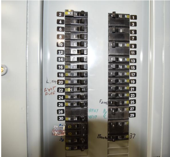
Fig.II.241 Interior view of panel and circuits breakers.
