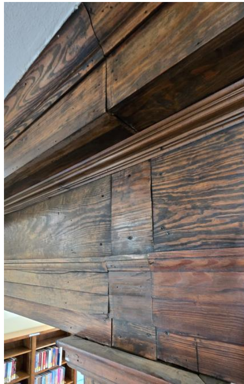
Fig.II.135 Southside beam shows extensive patching at old wall seam.
