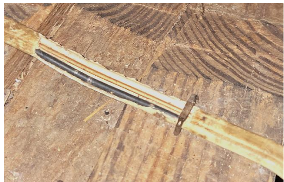
Fig.II.249 A small section of plastic-coated wire, located just inside the entrance to the historic attic, has worn away.
