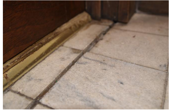
Fig.II.111 Water flows under threshold, collects inside and drains into wall cavity below.
