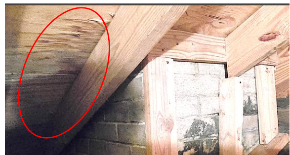
Fig.II. 73 Area below and adjacent to chimney cricket is currently dry but appears to have leaked in the past (red circle).
