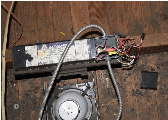
Fig.II.247 Many of the junction boxes on the HID ballasts are not properly covered.
