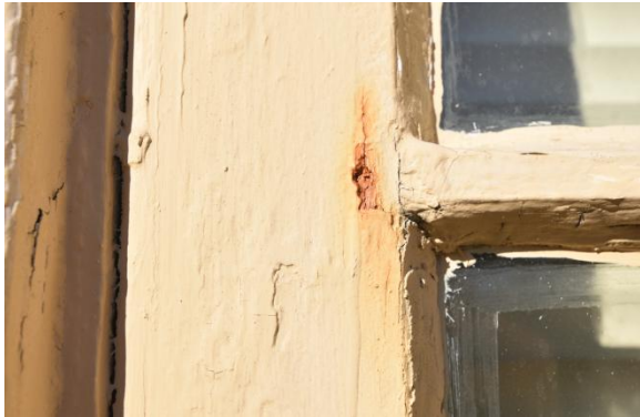
Fig.II.206 The window elements have good integrity but rust jacking was noted on several. Note the reddish stain where the muntin meets the stile.
