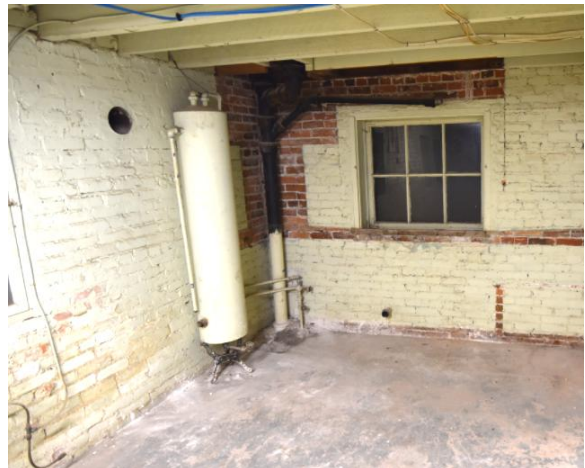
Fig.II.261 The antique hot water tank and plumbing stack are remnants of the original systems.
