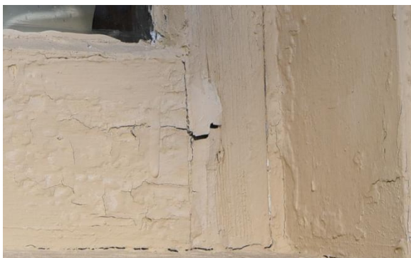
Fig.II.208 Several windows exhibited large chips or flaking.
