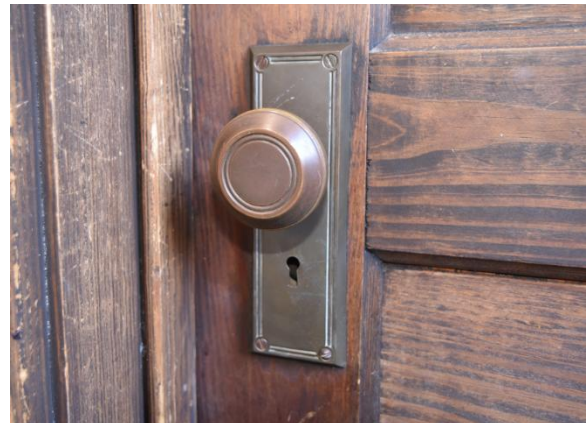
Fig.II.171 Original knob and lock mechanism in excellent condition.
