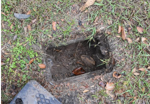
Fig.II.262 Water main hook-up inaccessible due to accumulated dirt and debris.
