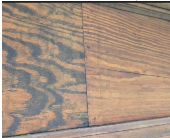
Fig.II.156 The wood on left is likely plywood made to look like the historic plank on the right.
