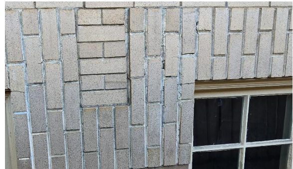
Fig.II.42 Failing mortar joints and material separation in water table on north elevation. Note: this may be related to the cracks on the interior walls along this same window.
