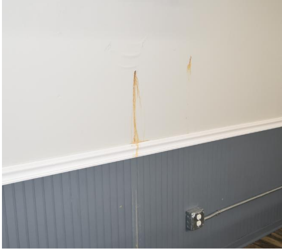
Fig.II.109 Rust stains are bleeding through from moisture trapped behind the wall board.
