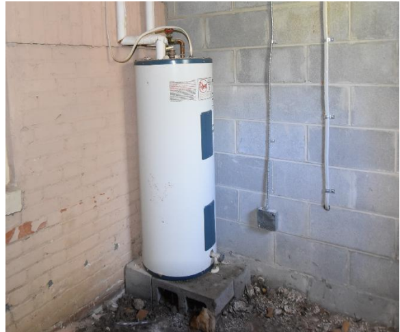
Fig.II.260 30-gallon hot water heater in basement.
