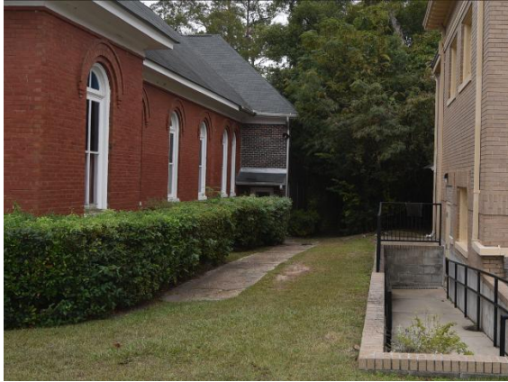
Sec. I/ Fig. 47 Concrete drainage apron between buildings likely not on library property.
