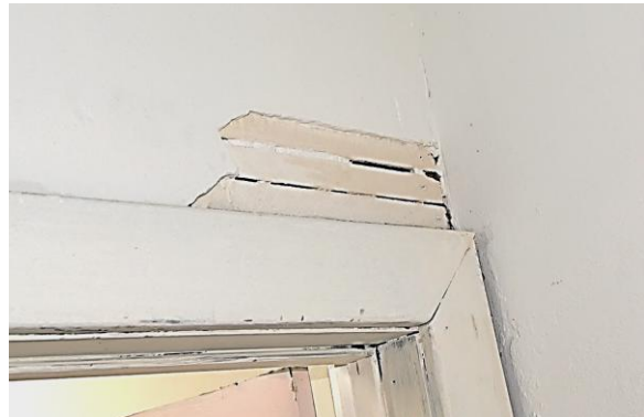
Fig.II.104 A damaged section of closet interior wall in the basement shows the wood lath that underlies the plaster.
