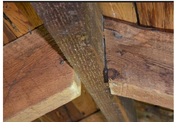
Fig.II.76 Rafter/ridge beam joint show minimal separation.
