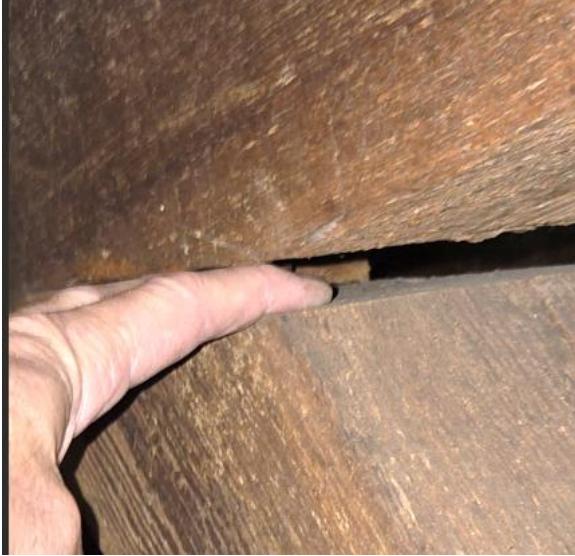
Fig.II. 77 The truss webbing has pulled away from the upper chord on both sides.
