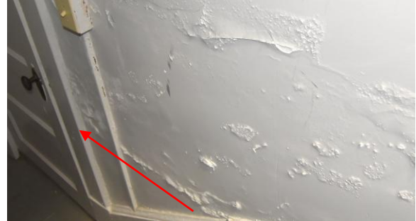
Fig.II.114 Note how the damage is spotty and in the lowest area, (red line) very horizontal. This may indicate the water is flowing along the internal mortar joints.
