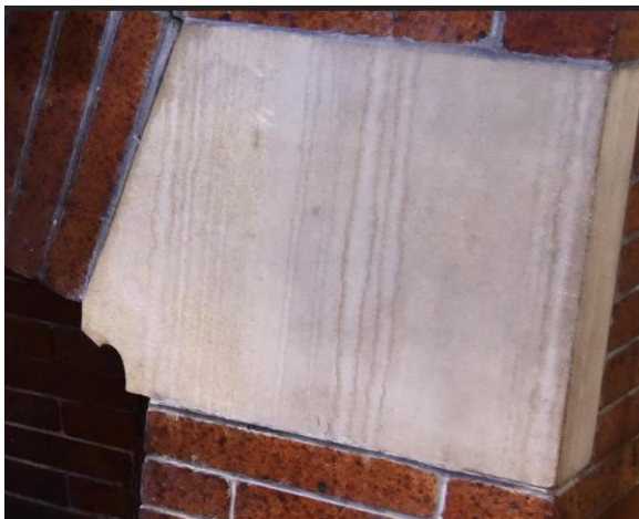
Fig.II.158 Water staining on northside fireplace.
