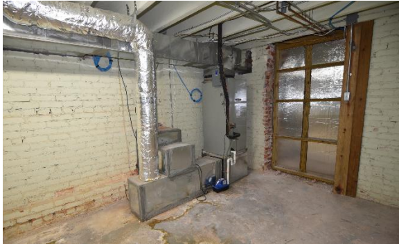
Fig.II.250 a 2.5-ton air handler cools the basement and rear rooms upstairs.
