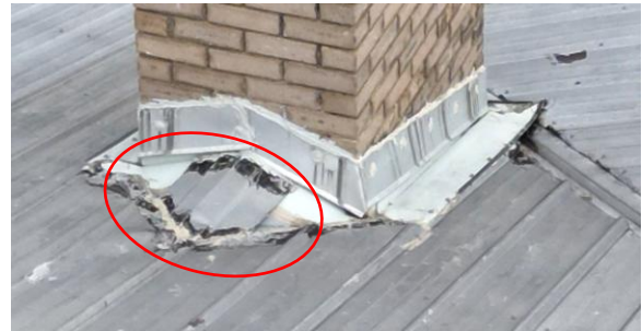
Fig.II.72 The cricket appears to have been patched several times after installation.
