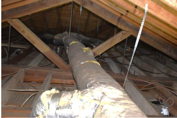
Fig.II.257 Air supply duct located in the historic attic.
