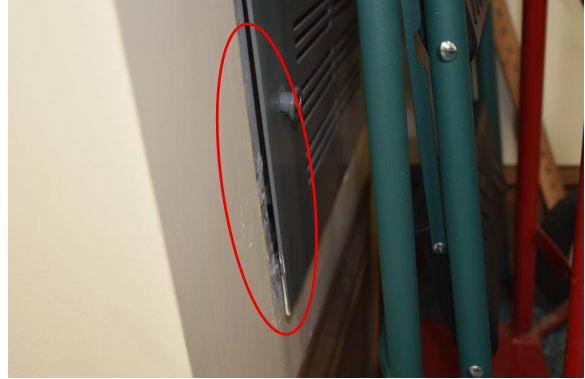
Fig.II.248 The lower portion of the main panel cover is loose.
