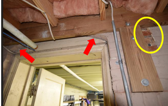
Fig.II.177 Note the obscured arch detail in the brick opening (red arrows). On right, an unpainted anchor area (yellow circle) for the shed roof that once covered this doorway.
