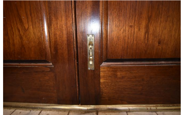
Fig.II.183 Lever on interior of main door is not operational.
