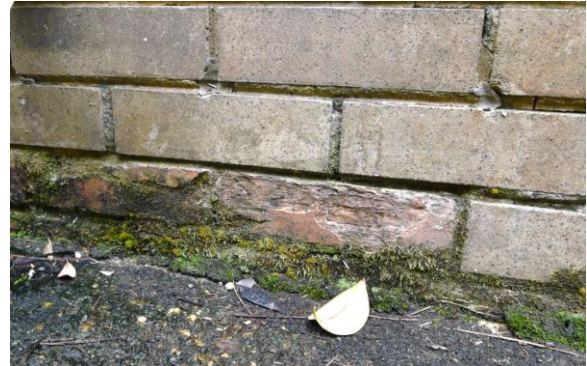
Fig.II.41 Spalling brick at grade on north elevation.
