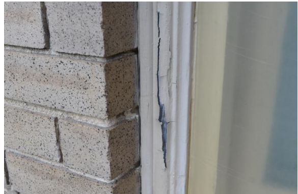
Fig.II.209 Some of the damaged areas are exposing the wood below which will lead to rot and deterioration.
