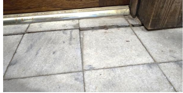
Fig.II.226 Note the damage grout and lowered tiles due to repeated water exposure.
