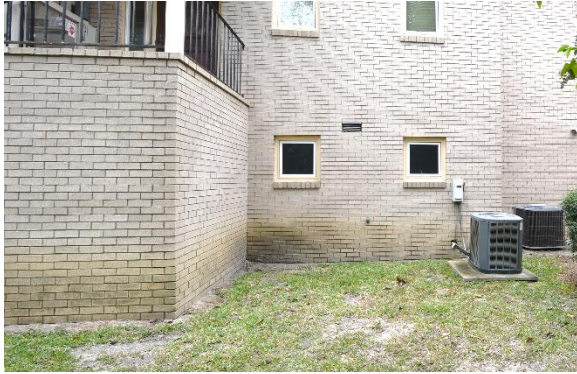
Fig.II.43 Lower wall staining due to moisture splashing back onto building during rain events.
