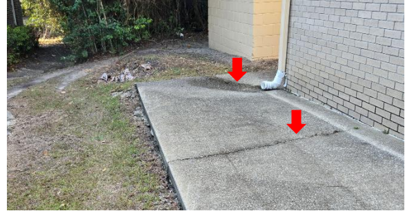
Fig.II.92 Poor drainage has undermined the concrete apron resulting in two full failures (red arrows) of the concrete slab.
