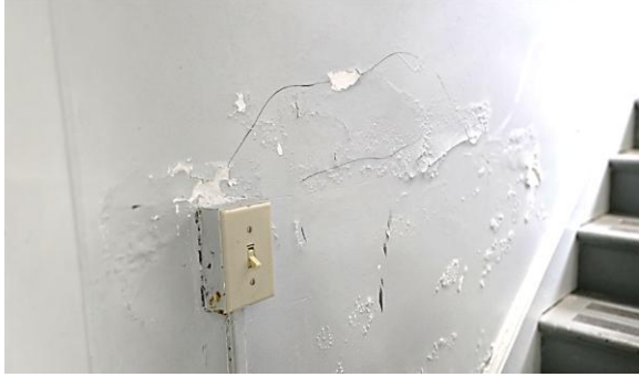
Fig.II.112 Extensive water damage to interior plaster finish in stairway.
