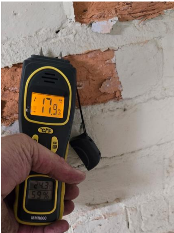
Fig.II.95 Moisture readings on the interior are very high.
