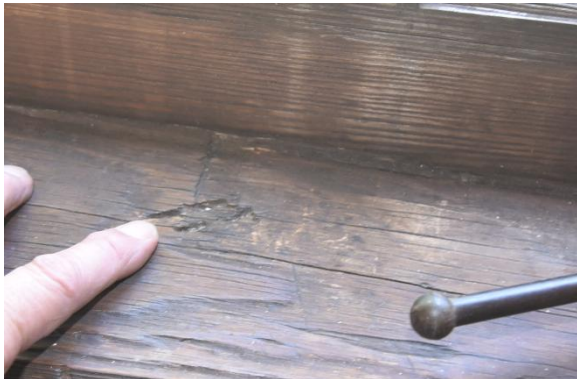
Fig.II.212 Some of the interior wood elements show past damage from water or sun.
