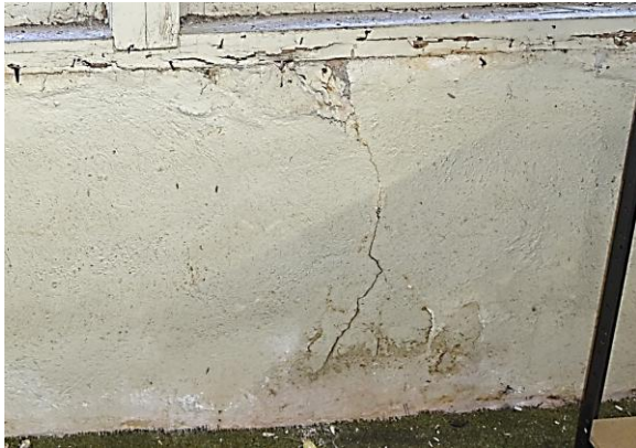
Fig.II.115 Water damage to interior wall along north side basement.
