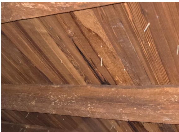
Fig.II.65 While some nail penetrations are visible, more would be expected given the multiple roofs the building has witnessed.
