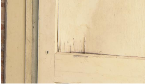
Fig.II.185 Broken upper panel on historic basement exit door.
