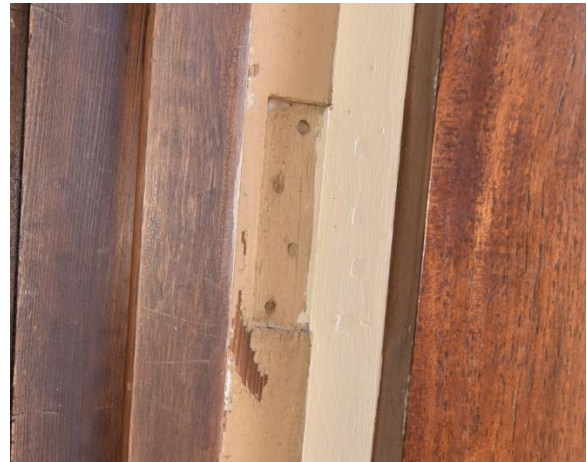
Fig.II.167 An earlier hinge mortise is visible in the jamb indicating a prior door mounting.
