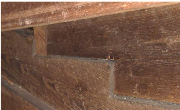
Fig.II. 78 The double notched heel joint appears well seated but may have shifted. Close inspection was difficult.
