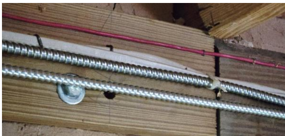
Fig.II. 243 There was limited use of BX/MC cable observed in the building.
