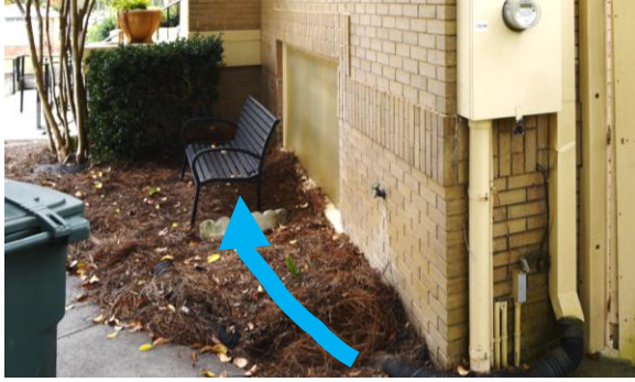
Fig.II. 94 Rainwater runoff is flowing down the slope toward the main entry wall and becoming trapped against the building.
