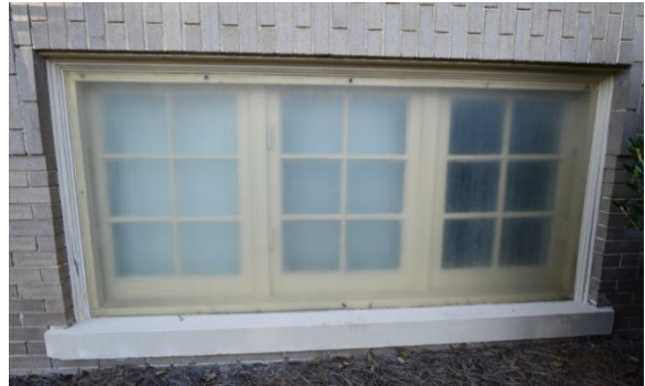
Fig.II.205 Plexiglass storm windows made front basement windows inaccessible for inspection.
