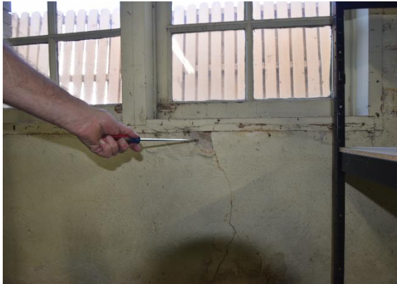
Fig.II.7 Failure in concrete skim coat below window may indicate foundational damage but likely caused by water invasion below sill.
