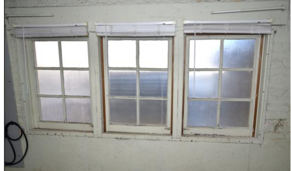
Fig.II.199 Windows in northside storage room have no interior trim.
