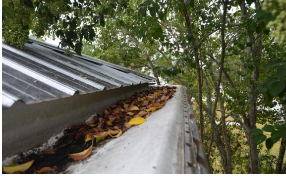
Fig.II.90 Upper elements of the drainage system need cleaning but are otherwise sound and operational.
