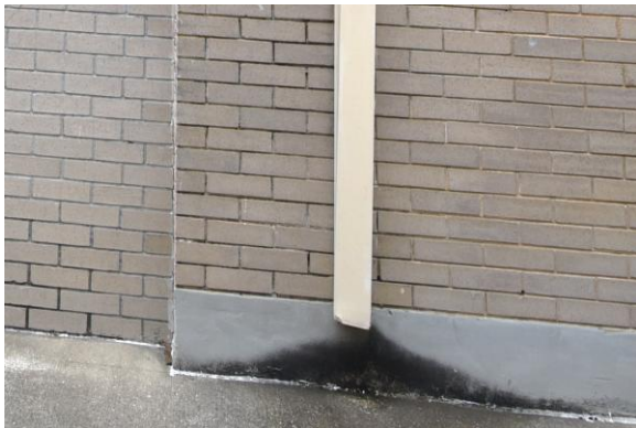
Fig.II. 91 Missing elbow and poor water drainage are undermining the concrete apron on the southwest corner of the building.
