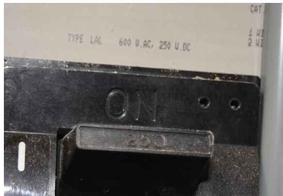
Fig.II.240 Main break indicates 250 amps of service in the building.
