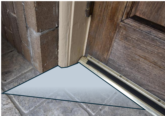
Fig.II.110 During rain events, water is pooling up on the outside of the threshold because the stoop is slope down and inward here.
