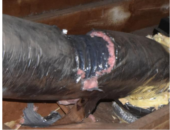
Fig.II. 79 Damage from critters to HVAC duct insulation, probably squirrels, was observed in attic.
