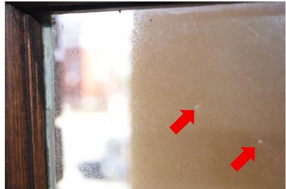
Fig.II.195 Some of the glass shows signs of its early manufacturing process. Note the pits in this entry window.
