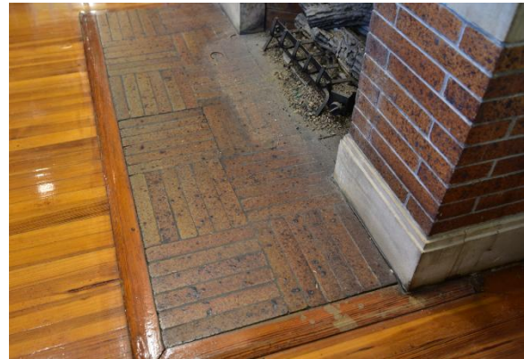
Fig.II.147 Broad hearth allowed fireplace to be functional.
