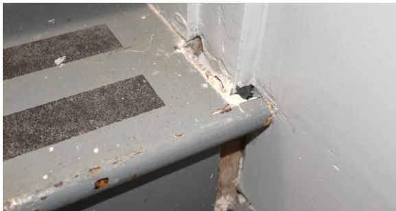
Fig.II.234 Evidence of a notch, perhaps for a newel post that was originally anchored at this spot.
