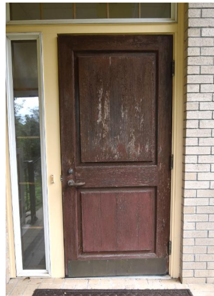
Fig.II.184 Exterior rear door needs refinishing.
